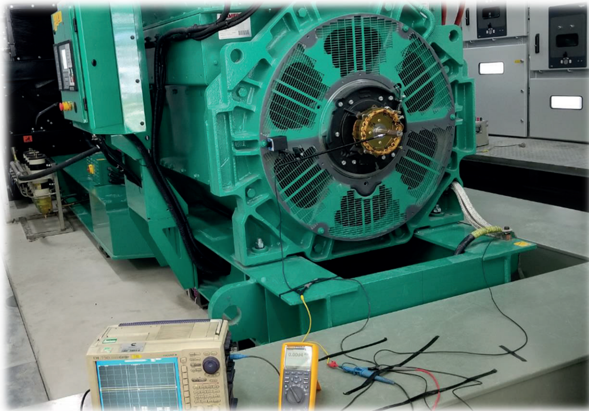
Figure 1: HVSI804S1 Alternator with Shaft Voltage testing apparatus
