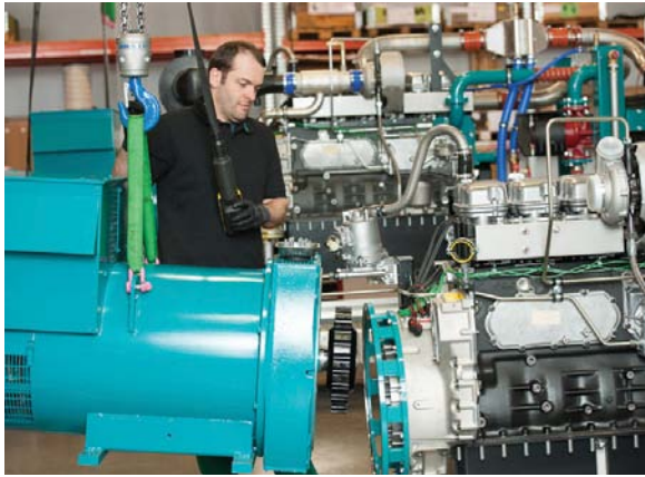
Coupling the STAMFORD generator to the engine at SCHNELL's headquarters in Amtzell, Germany
