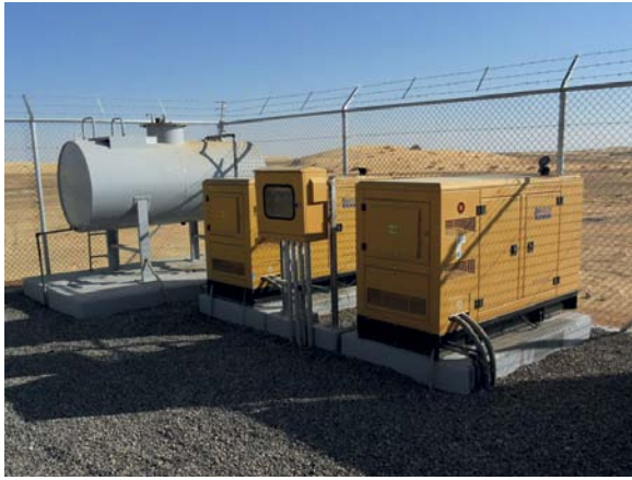
Shanghai Cooltech Power's generating sets with STAMFORD P1 generators in situ
