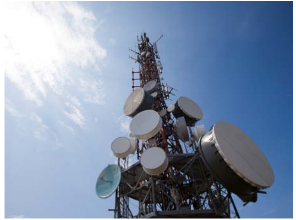
One of the 300 base stations deployed in Saudi Arabia
