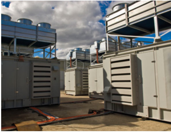
Generating sets ready for shipment to Barrow Island from MPower's Ingleburn facility
