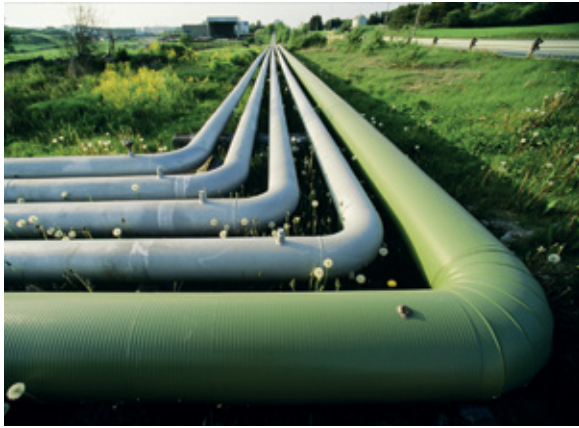
Gazprom rely on dependable power for delivering gas to customers through 1,500 km of pipelines
