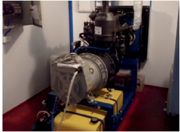
STAMFORD P1 alternator in operation providing critical power to Gazprom's oil and gas project
