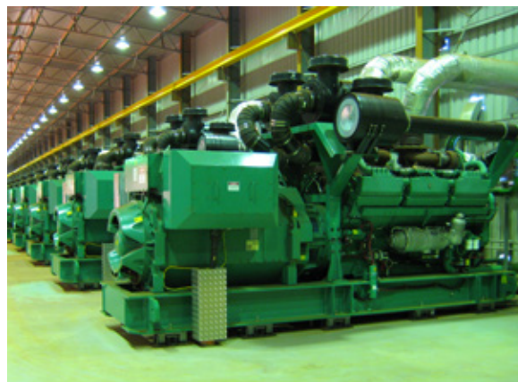
28 high voltage STAMFORD P80s were specified for the generator sets
