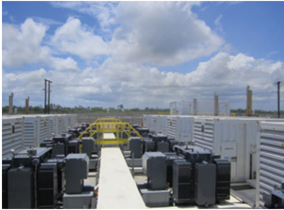
30 x 1,250 kVA generator sets power the site
