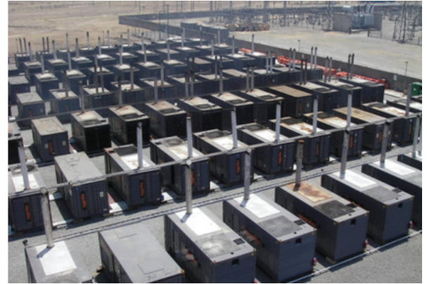
Figure 1: A Typical Power Plant made of smaller Gensets.
